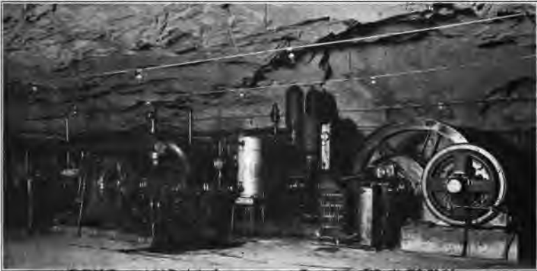
UNDERGROUND PUMP AT THE GWINN MINE
